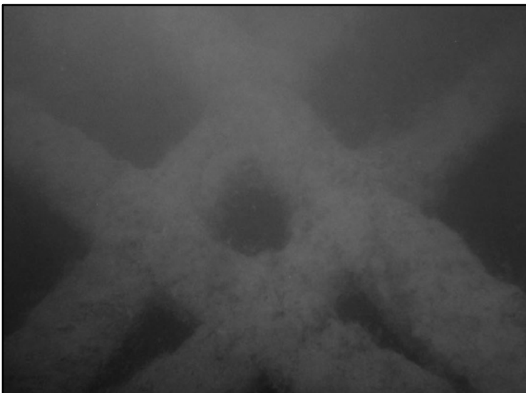
Covered with silt and algae growth, cross work of the collapsed suspension bridge tower, submerged since 1936. (Photos: Robert Cornellier, 2012)
